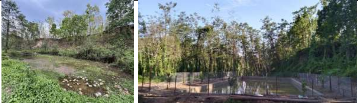
Fig. 1: Construction of fishery pond in Ghagar sub-watershed, Kamalamai Municipality-1, Thunuwa, Sindhuli (Left: Before intervention; Right: After intervention)
